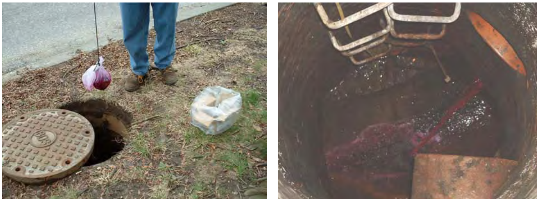
Figure 64: Dye in a mesh bag is placed into an upstream manhole (left); Dye observed at a downstream manhole traces the path of the storm drain (right)
