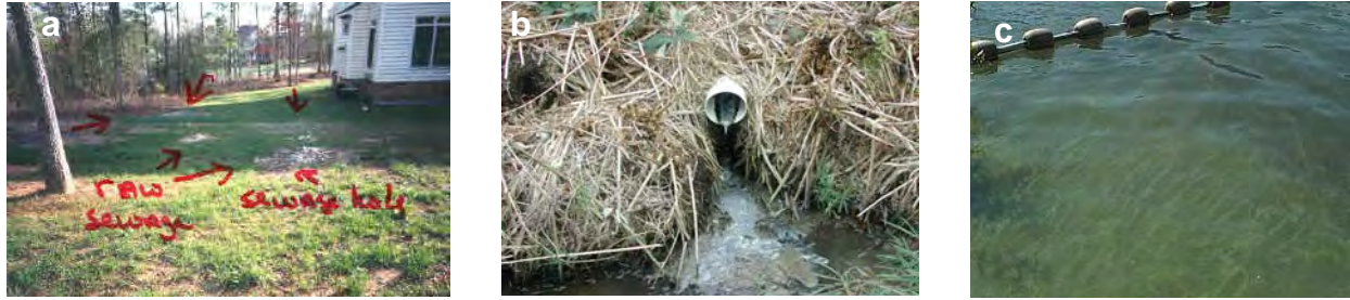
Figure 72: (a) Wet, spongy ground. Grass may be bright green or burnt due to high nutrient loading. (b) Straight pipe discharge to nearby stream. (c) Algal bloom in a nearby pond.
