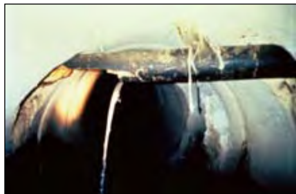
Figure 1: Sewer Pipe Discharging to the Storm Drain System
